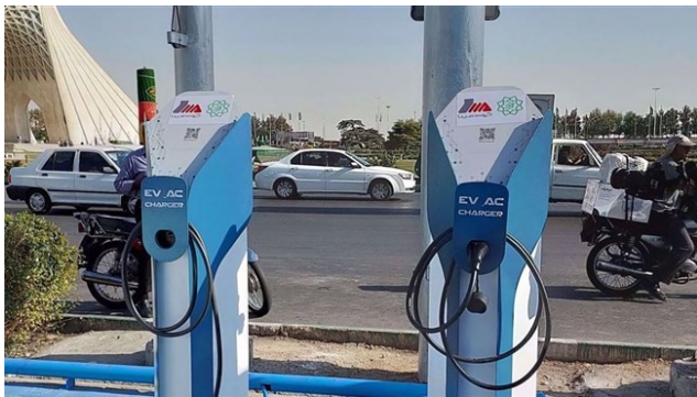
Fig. 3. View of a charging station installed in Tehran [26].
